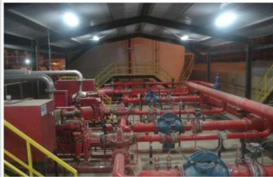
VTTI Kenya, firewater pump hose, firewater system designed to NFPA standards
