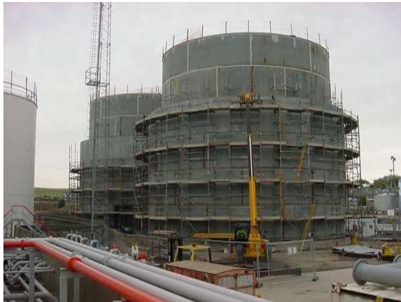
Aberdeen Terminal, Scotland - New double walled Tankage under Construction for BP Exploration.
