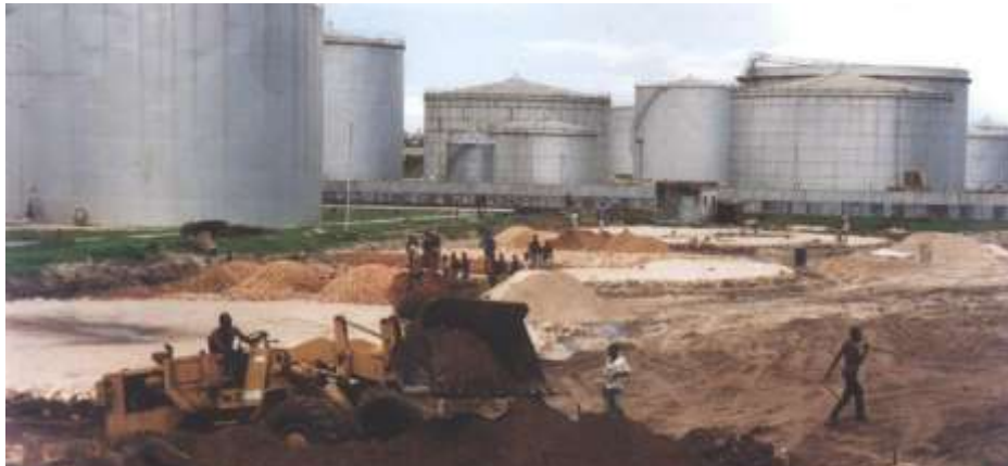
World Bank funded Marine Oil & Gas Pipeline Reception Facilities and Cross-country Pipelines Project Management by BP Tanzania Design by Trident Engineering Consultants.
