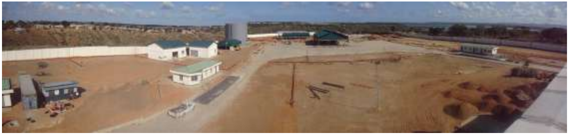
New LPG storage and distribution terminal receipt from off-shore CBM Currently under construction, commissioning planned Jan 2013.
